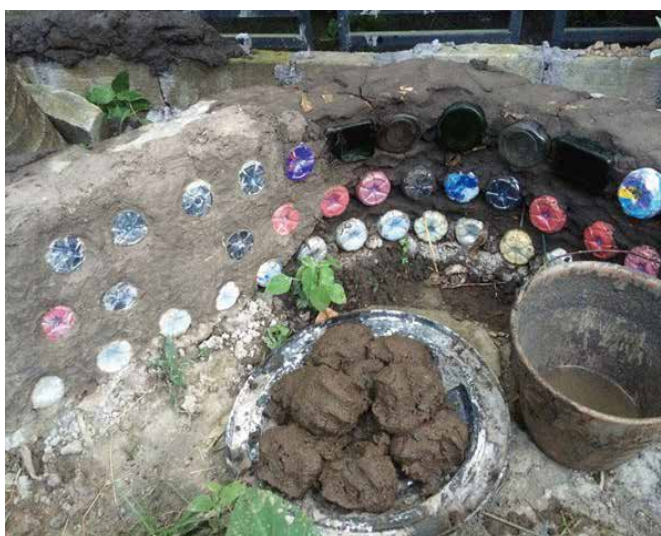
▲ Figure 2 : Global Ecobrick Alliance building a wall with EcoBricks using cob, a natural building material, to bind the EcoBricks together. https://www.ecobricks.org/earth-methods/
